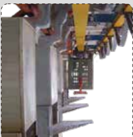
Automatic portering system (central furnace)
